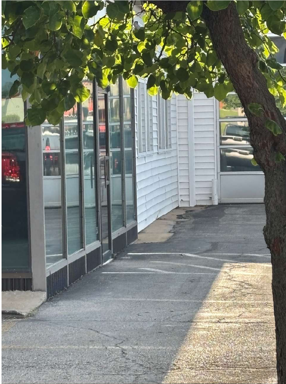
Figure 7. Unauthorized parking stall lines remain in front of building entrance. 8-28-26
